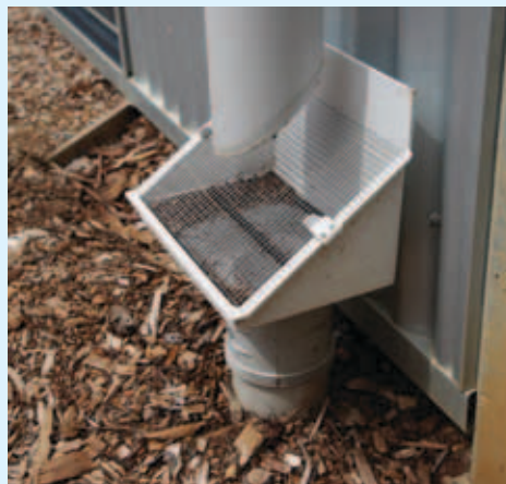
↑ Leaves and other debris washing out of the box gutters are shed by angled mesh inserts in the downpipes, minimising maintenance. The captured rainwater is passed through another finer filter before it enters the tanks. Photo by Anna Cumming
