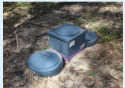
↑ All waste water is treated on site. Currently it's used only to water the garden, but the infrastructure is already in place to use the recycled water in the laundry and toilets when legislation permits. Photo by Anna Cumming
